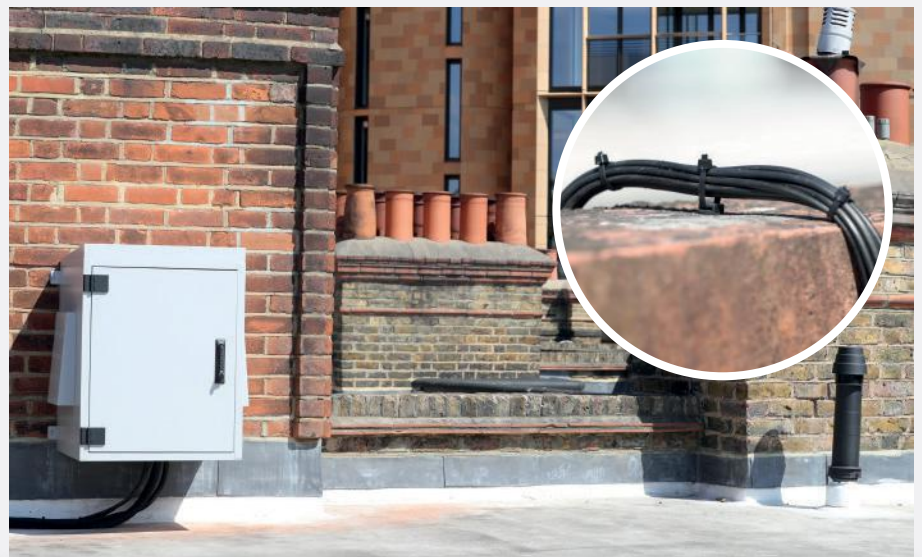
Cabinet located on the roof of the development with neat cabling
