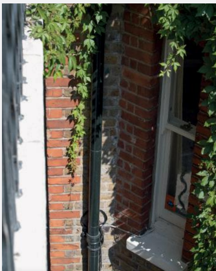
External cabling concealed behind pipes
