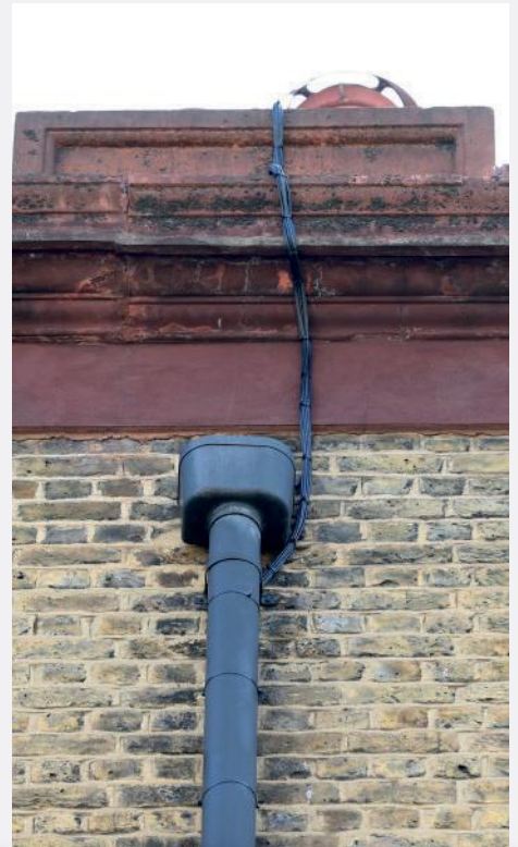
Cabling from roof to external walls
