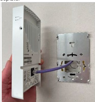
The cable is plugged into the back of the H550
